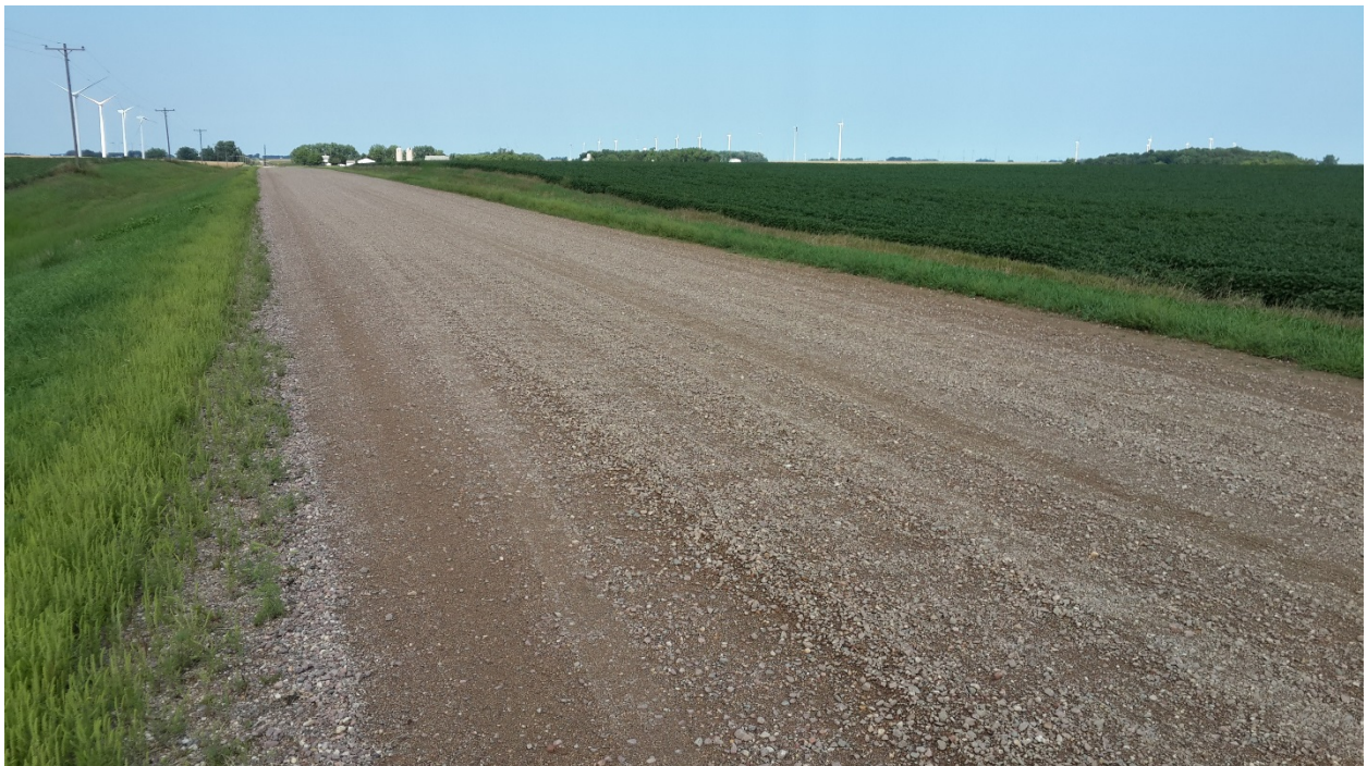
Figure 22 Jackson County Road 76 Surface Conditions in August, 2013 (Photo by the Author)
