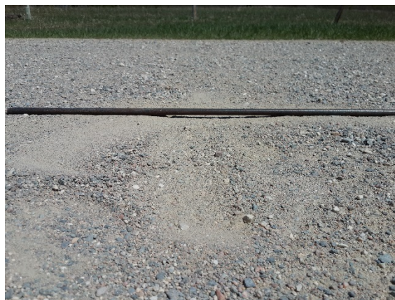
Figure 61 Typical Corrugation in the South Section/3 rd Section (Photo by the Author)
