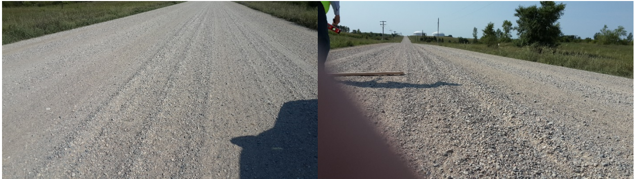
Figure 3 Loose Aggregate on CR 35, Pope County, July, 2013 (Photo by the Author)
