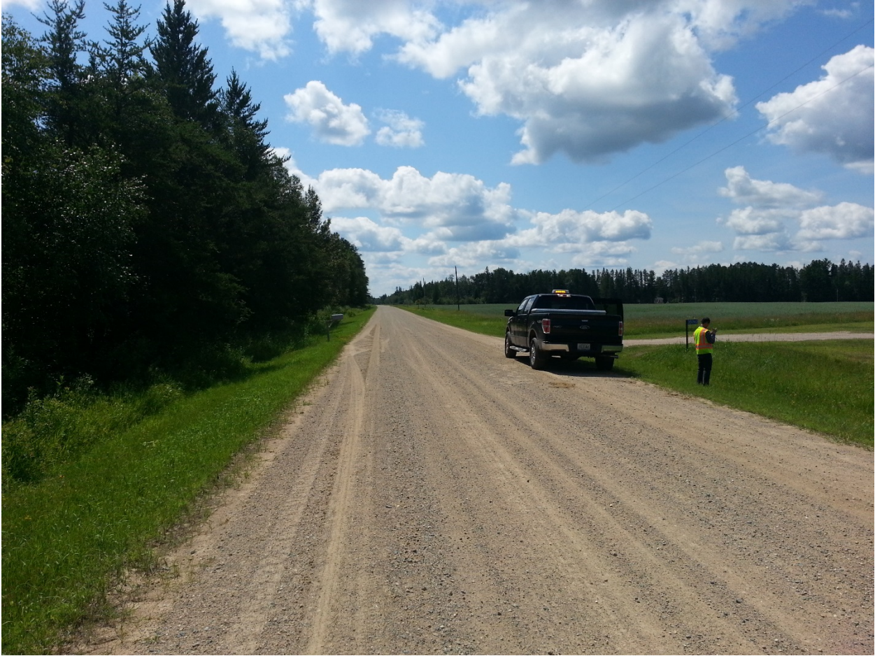
Figure 23 Beltrami County Road 23 Surface Conditions in July (Photo by the Author)
