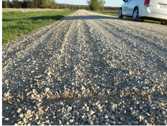
Figure 71 Loose Aggregate on the Surface of Section 1
