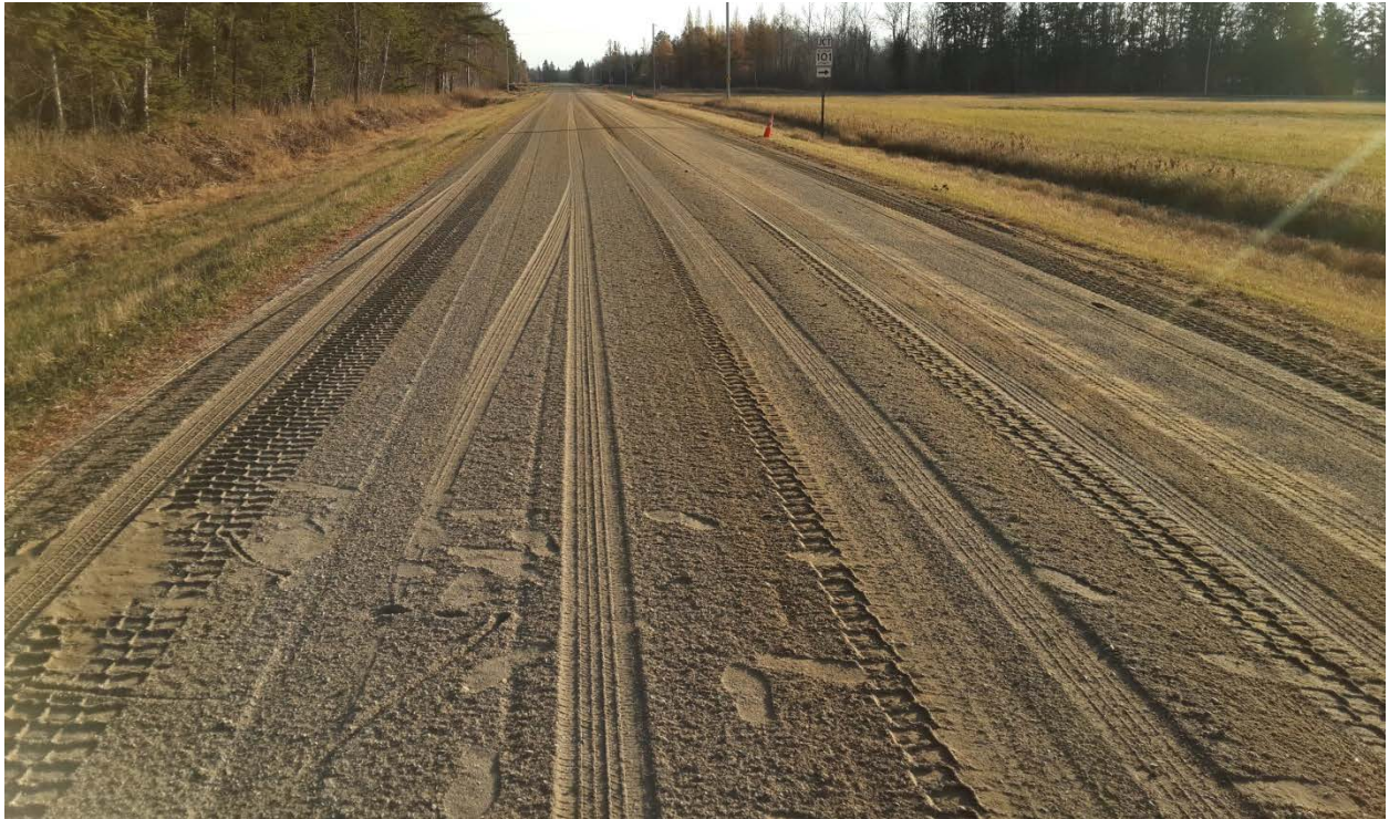
Figure 32 Beltrami County Road 23 Mid Test Section (Photo by the Author)
